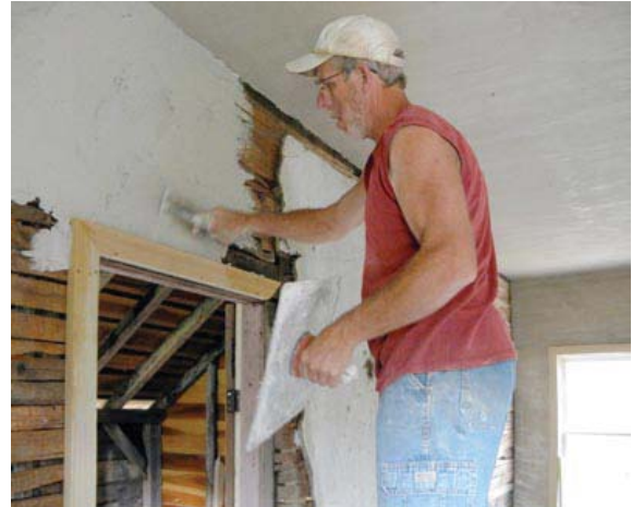
Terry putting on the scratch coat of plaster. The final surface was a thin lime coat, painted on, duplicating the original finish.
